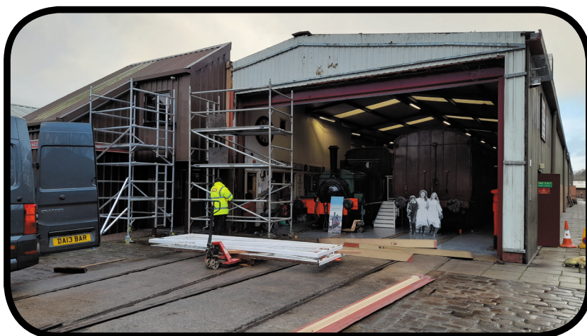
Preparation for the recladding of the front of the Museum January 2023 - Photo: Paul Holroyd
